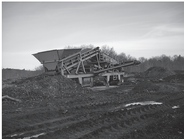
FIGURE 8.4 Composting equipment and windrows town of Glenville, NY. (Courtesy of town of Glenville, New York.)
