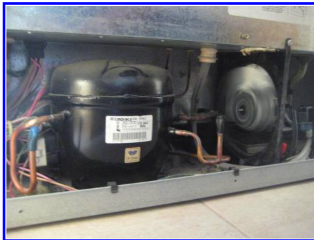
Figure 4.6: A typical compressor and cooling fan next to it.
