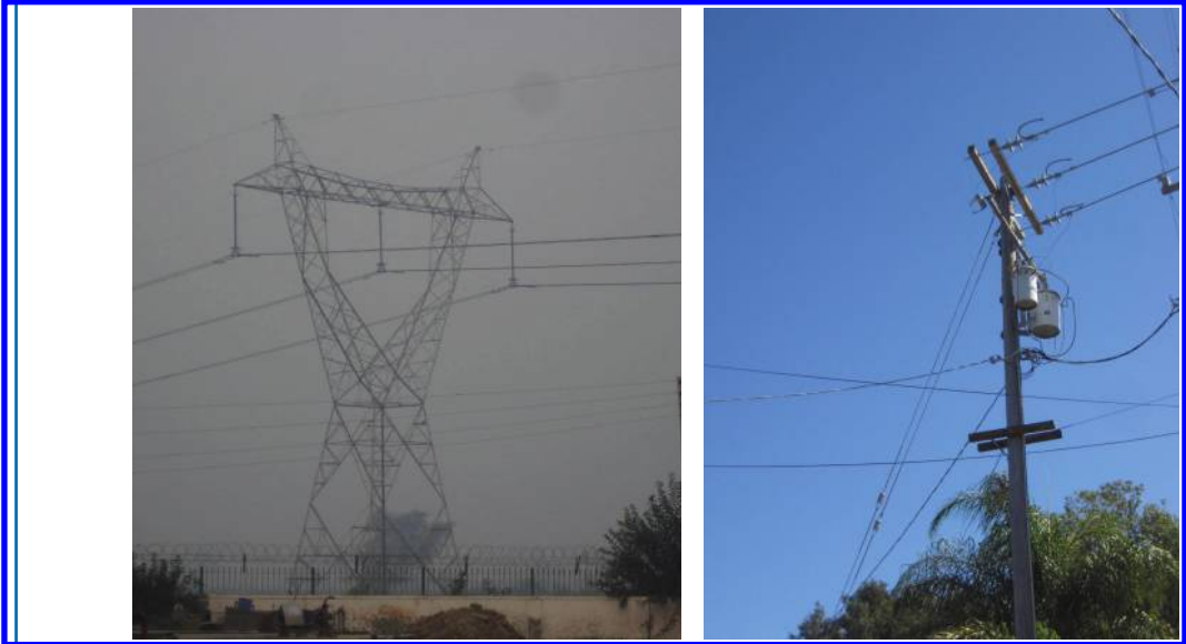
Figure 6.24: Typical transmission lines and transformers on power poles that reduce electric power from tens of thousands of volts to 110 volts for domestic consumption.
