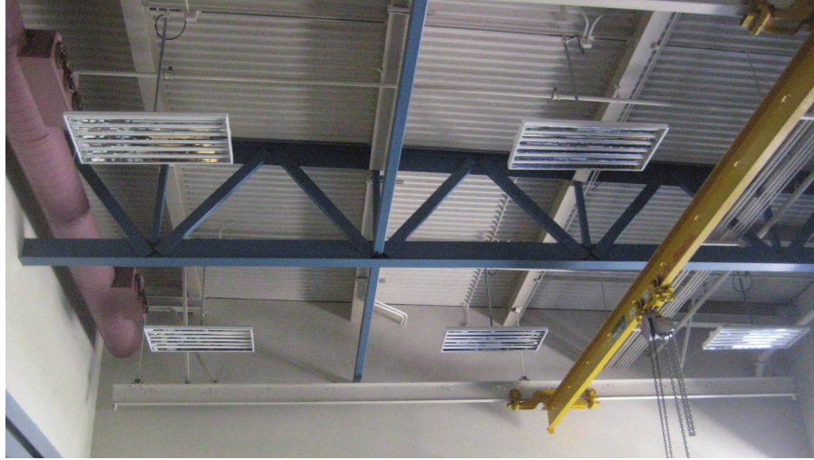
Figure 5.12: A truss used as a load-carrying element in a ceiling. The second moment of the area of the truss is significantly larger due to the way the elements are distributed farther away from the neutral axis.
